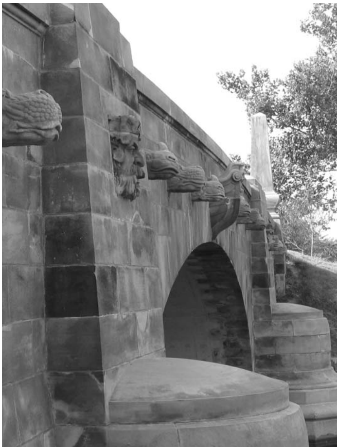
The Lake Shore Drive reconstruction work on Chicago’s South Side is a prime example of applying context sensitive design principles.
